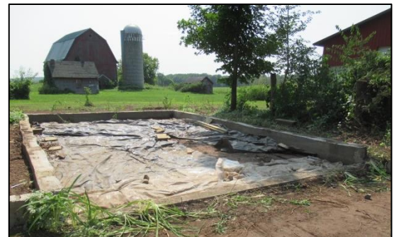
Leaving nothing behind except an empty foundation that had served its purpose since 2003.
