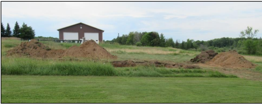
Mid July an excavator was hired to prepare the new location. Top soil was pushed aside and the proper sized hole was made in the SW corner of our lot.
