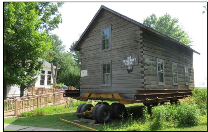
Once the building was safely and securely attached to all the wheels, it was pulled off of its location and parked next to German Settlement Road....ready to be hauled away.
